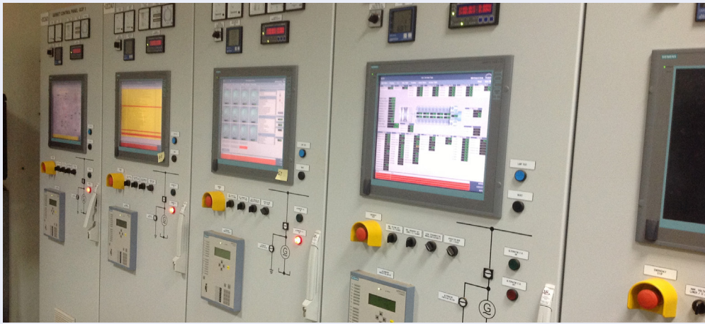
Thika power plant control room.
